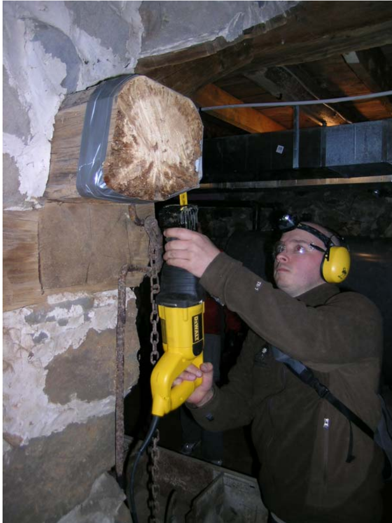
Figure 2.0: The end piece of a log (Mad Lab # 07CS001) built into the fireplace that was used in the analysis of the Lowden House.
