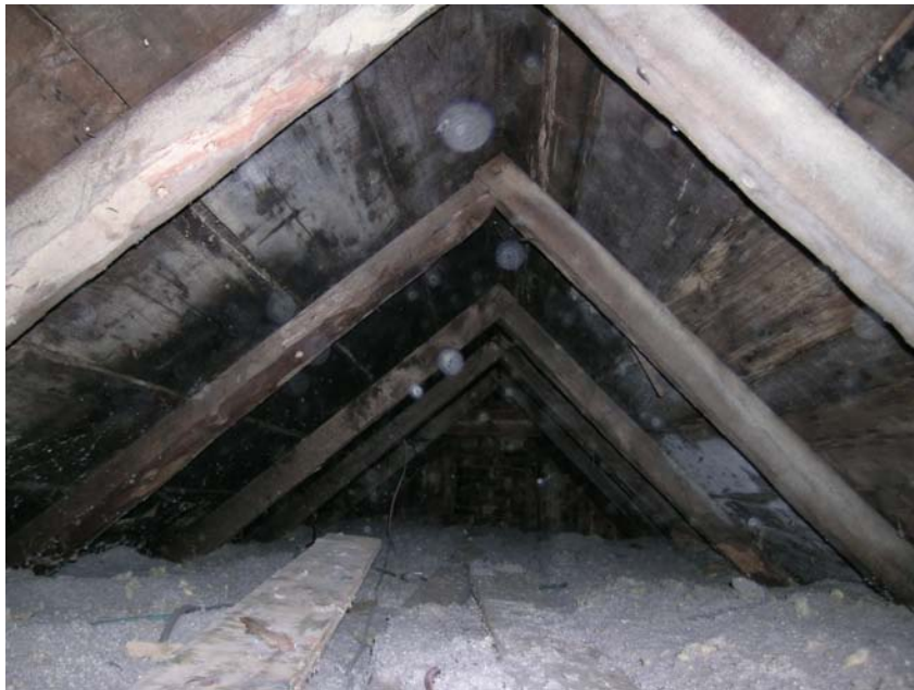
Figure 1 - A view looking down the attic space above the older part of the house. The rafters in this section of the house were pegged together with wooden dowels and the beams were both sawn and rough hewn.
