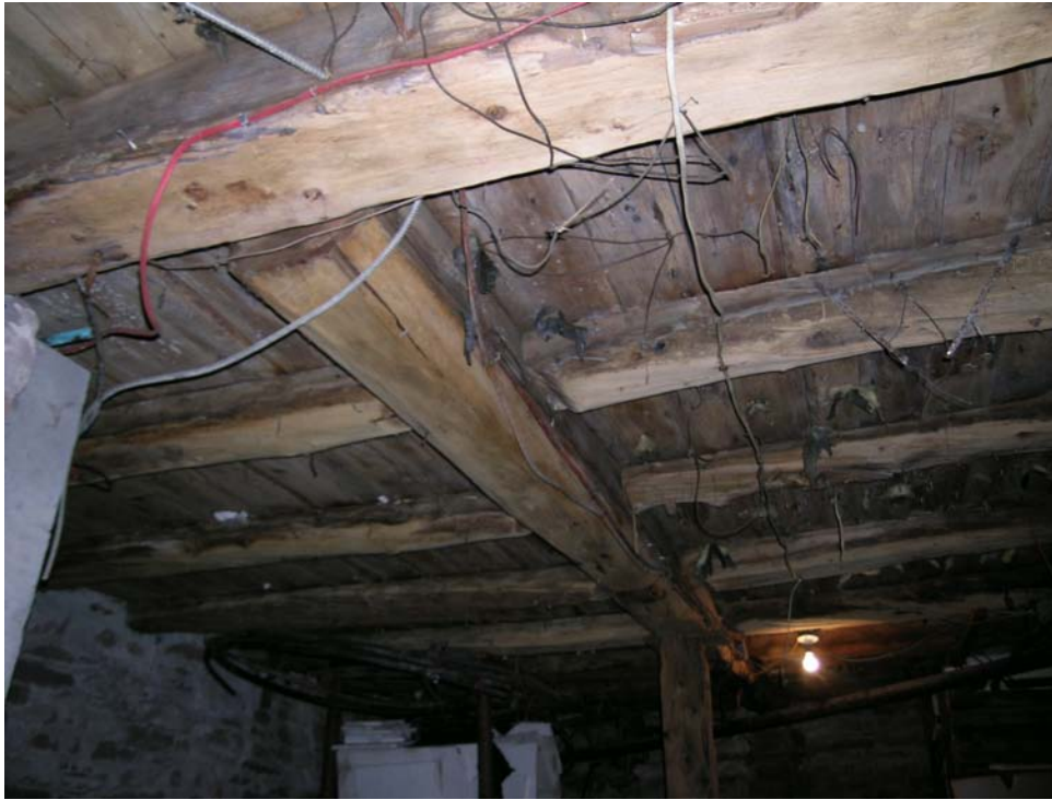
Figure 2 - A view of the basement beams below the older part of the house. The beams in this section of the house were notched together and flattened in places by an adze.
